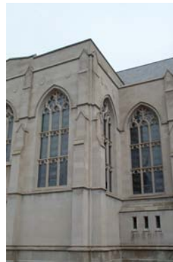
Figure 8: An image of a church facade captured with the world and camera coordinate frames as described in Section 4.5. The vertical vanishing point is forced to fall on the image y -axis. Also, the horizon is forced to be parallel with the image x -axis.
